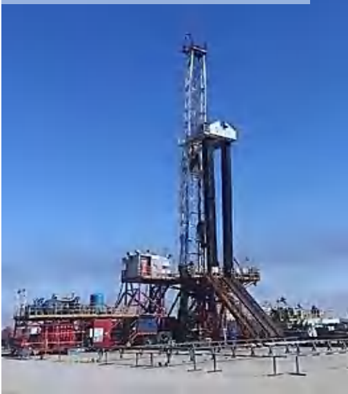
750HP Workover Rig
